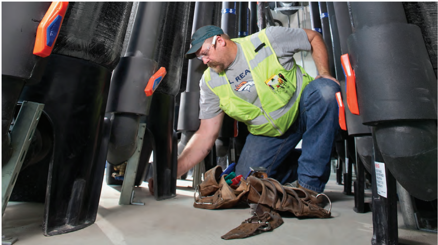
A Watts OneFlow® antiscale system installation.
