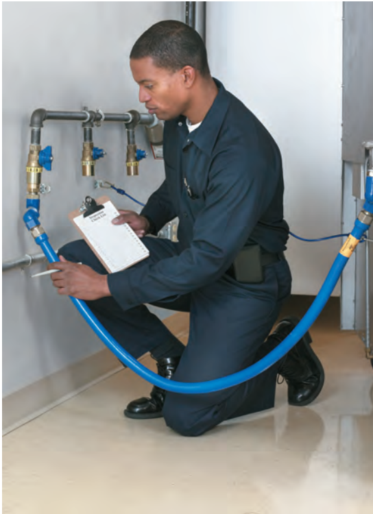
A Dormont blue hose gas-connector installation in a commercial kitchen.
